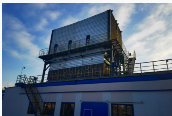
空压制氮干湿联合冷却塔
