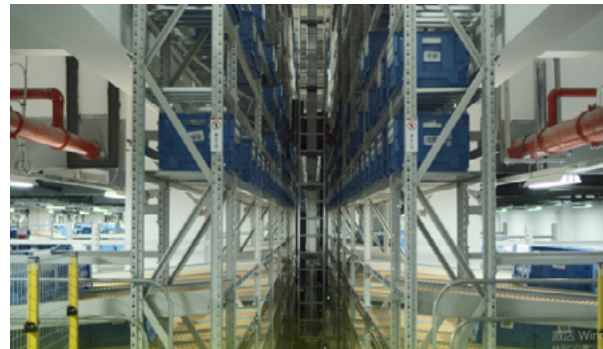
Minload Intelligent Automatic Replenishment System
