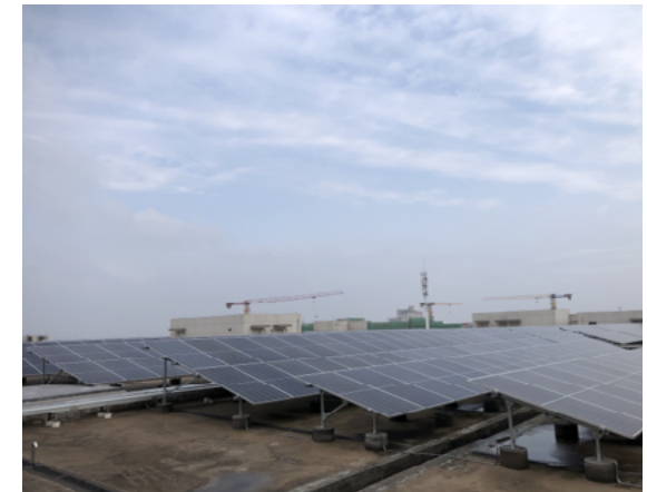
The Photovoltaic Power Generation Project in Jiangxi Yifeng Pharmaceutical Industrial Park
