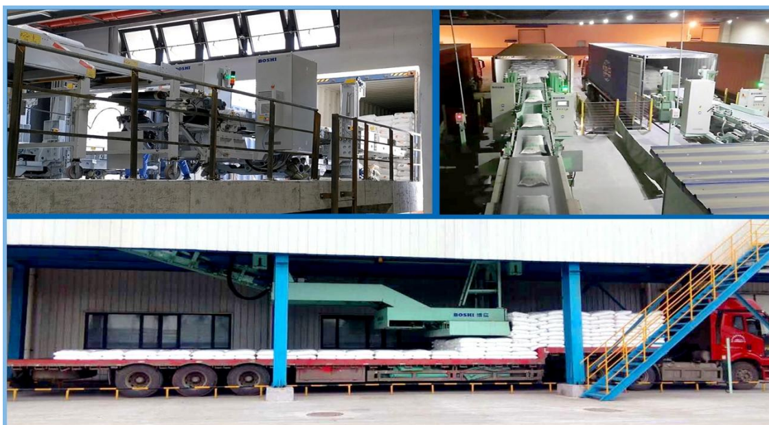
Legend: Partial photos for automatic vehicle loading system
