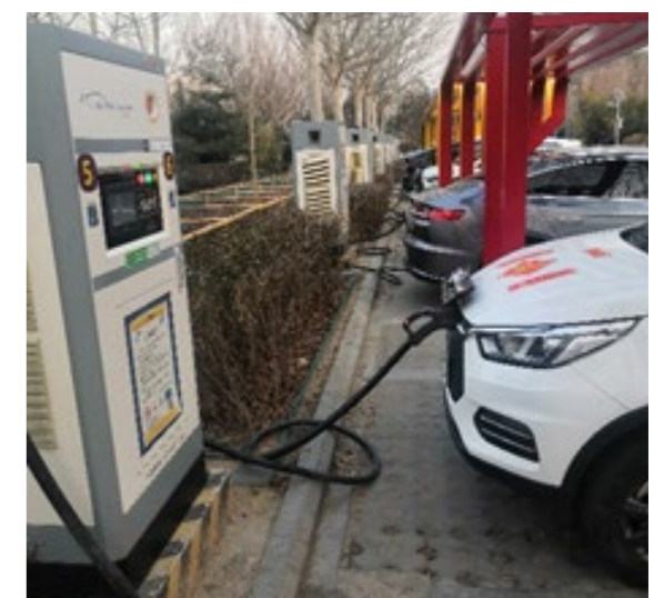
Charging piles around TransInfo Building
