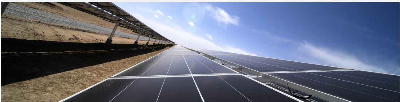
Photovoltaic composite project in Majiatan, Lingwu, Ningxia
