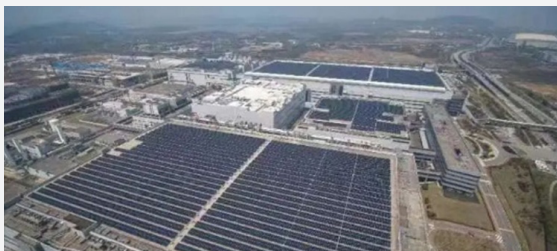
Wuhan Huaxing rooftop-distributed photovoltaic power generation project
