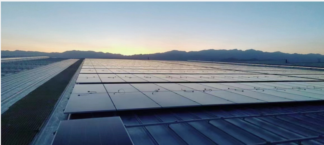
Distributed photovoltaic project at Ningxia-Zhonghuan Industrial Park
