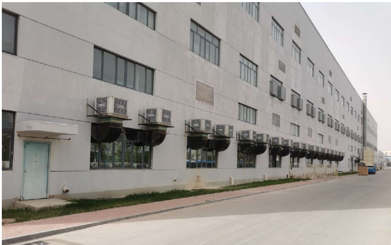
(图为水冷空调及排潮风机)
