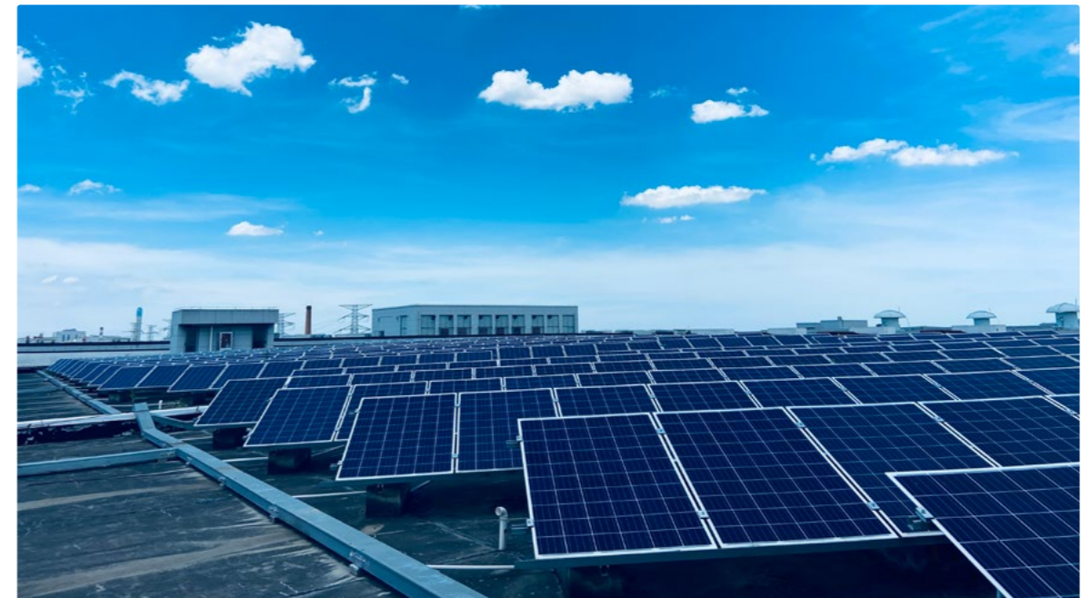
The Photovoltaic System Located on the Rooftop of the Second Floor in the Longshan Base Center of the Company
