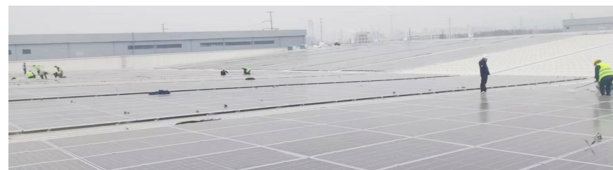
Rooftop Photovoltaic Installation
