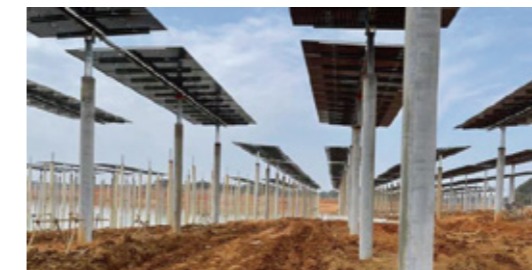
Fishery and Light Complementary Solar Power Station
