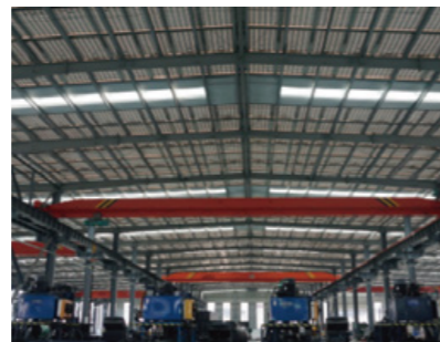
Inside the BIPV roof of the plant
