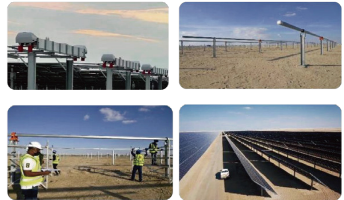
PV Plant in the Abu Dhabi Tracker Application Project
