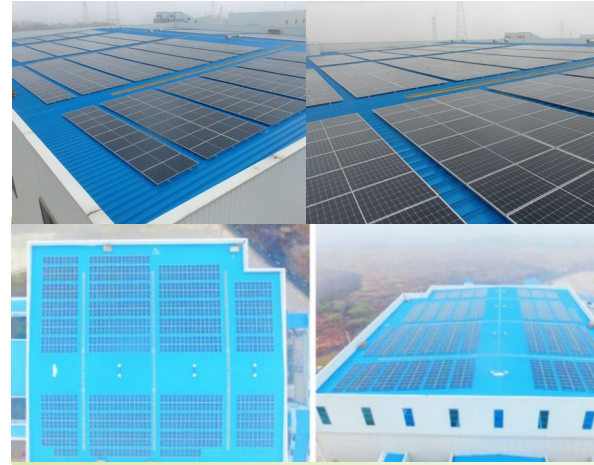
Aeroview of the 2.5 MW photovoltaic power generation project at Hunan Jiuhua
