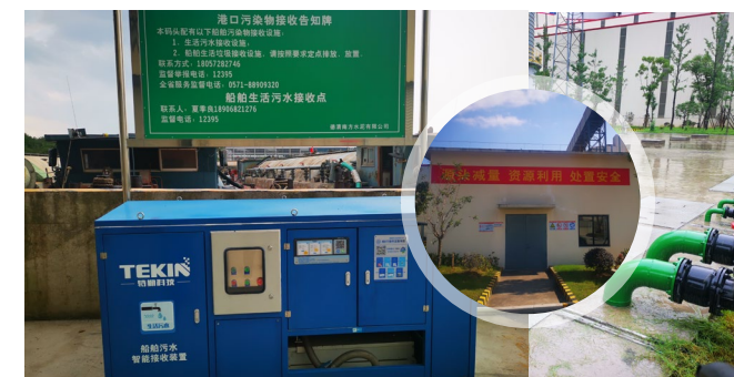
Deqing South's water treatment system
