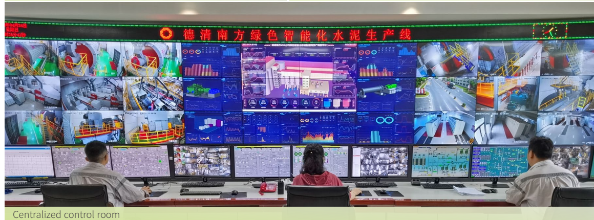
Centralized control room
