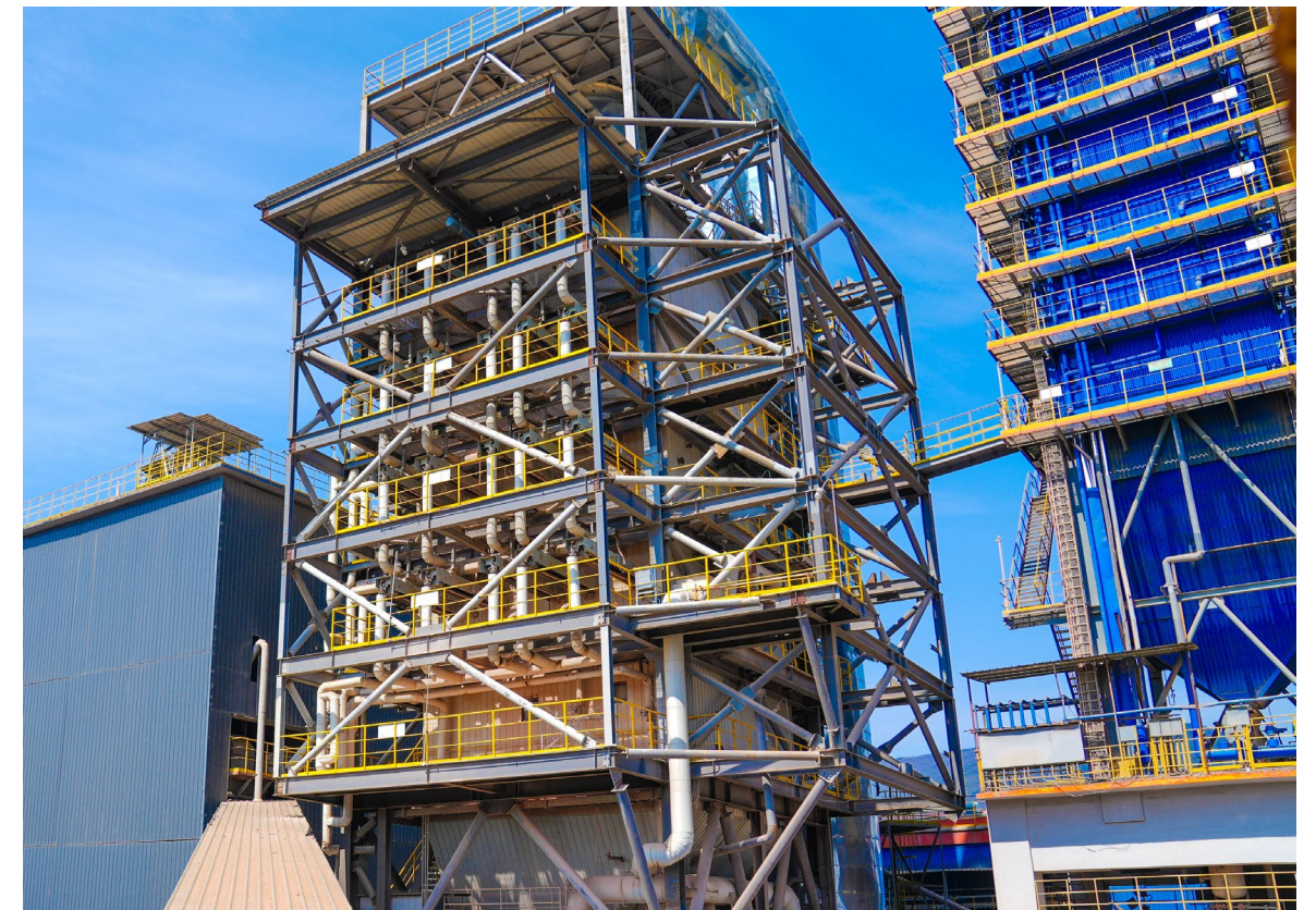
Changxing South's SCR denitrification project for exhaust of kiln tail in clinker line
