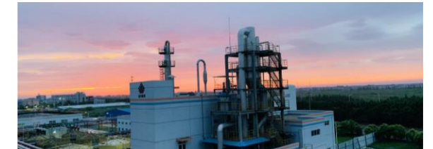
● Ammonia distillation tower of a factory
