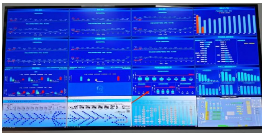
智能温度监控系统监测大屏
