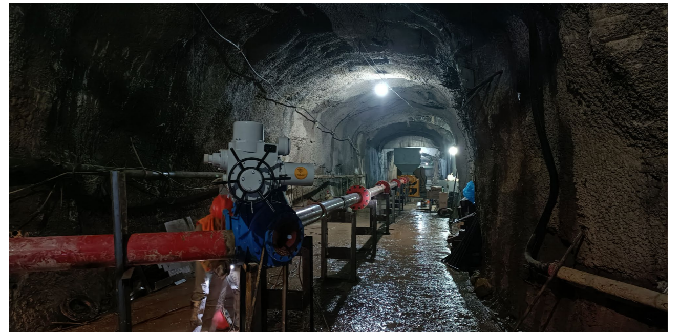
Tailings paste filling pipeline
