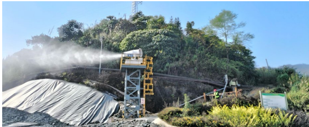
Spray dust suppression device in the Daping beneficiation workshop of Hualian Zinc and Indium
