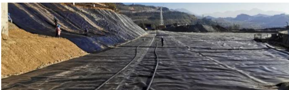
Impermeable membrane is laid in the raw ore storage yard of Hualian Zinc Indium Daping Workshop
