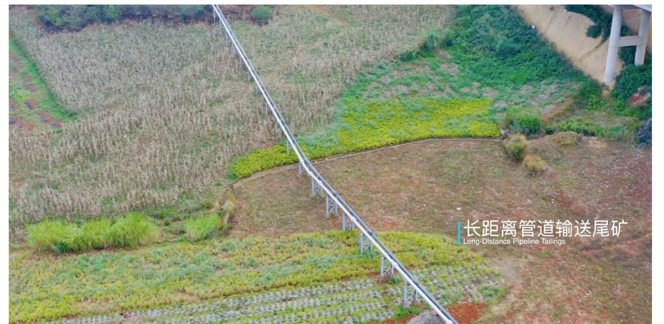
Tailings transport by long-distance pipeline
