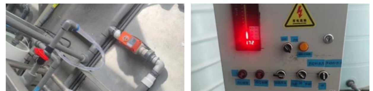
New waste water treatment equipment
