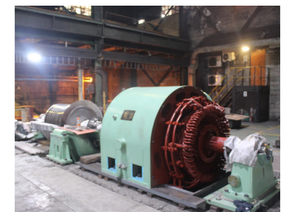
Newly Built Waste Heat Turbine Generator at Smelter
