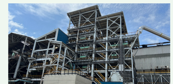
New DSB Furnace
