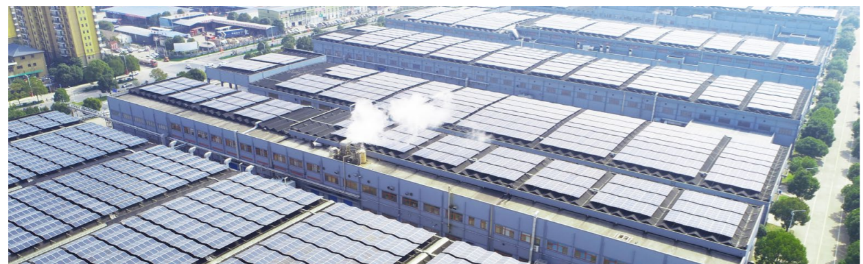
Photovoltaic Panels Installed by the Company
