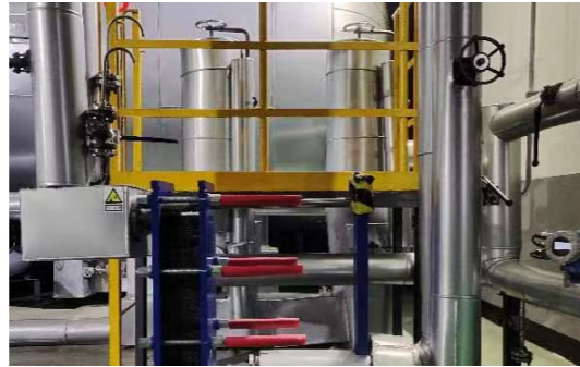
Waste Heat Utilization of Condensate Water of S Line
