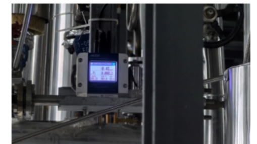
Realistic View of Small-flow High-precision Control Project after Transformation
