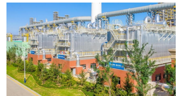
Seawater Desalination Plant
