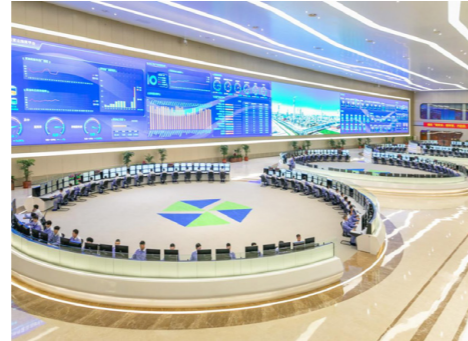
Central Control Room
