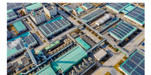
Construction of Solar Photovoltaic Power Generation on the Roof of the Plant
