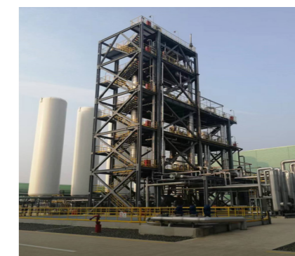
Carbon Dioxide Recycling Unit
