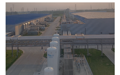
Environmental protection facilities at Suqian Optoelectronics production base
