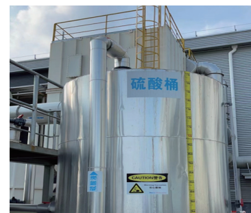
Sulfuric acid dosing device for acid absorption at Yancheng Technology base
