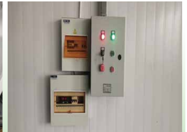
Pollution control location: Adjacent to the bonding room
