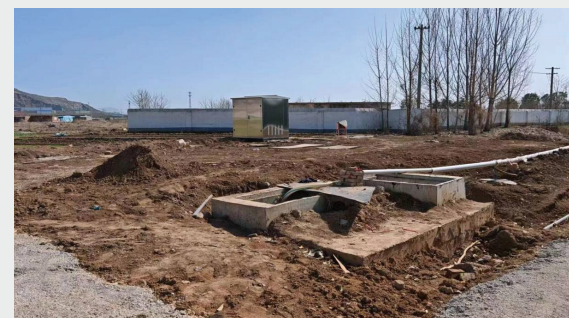
Integration Project in Zhang Village, Sili Town (Treatment Capacity: 150 m 3 /d)
