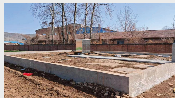
Integration Project in Libazhuang Village, Chengliu Town (Treatment Capacity 50 m 3 /d)
