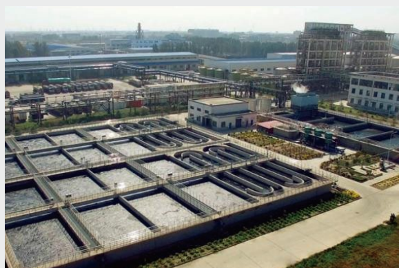
Jinkai Synthetic Ammonia Sewage Treatment Plant with an Annual Capacity of Millions Tons (Treatment Capacity: 20,000 tons/day)
