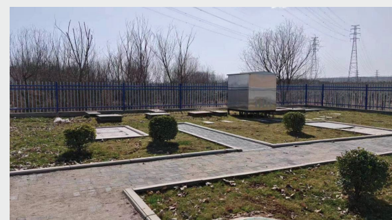
Integration Project in Yuyang Village, Sili Town (Treatment capacity: 100 m 3 /d)
