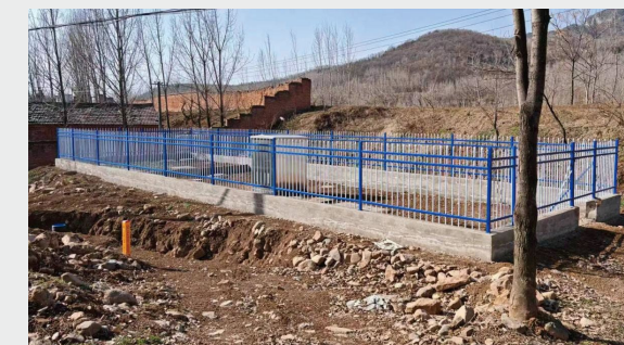
Integration Project in Xiashenmiao Village, Sili Town (Treatment Capacity 50 m 3 /d)
