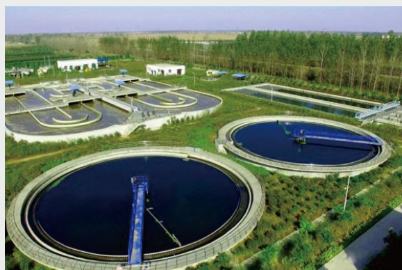
Sewage Treatment Plant in Songjiang Industrial Cluster Area in Luohe City (Treatment Capacity: 30,000 tons/day)
