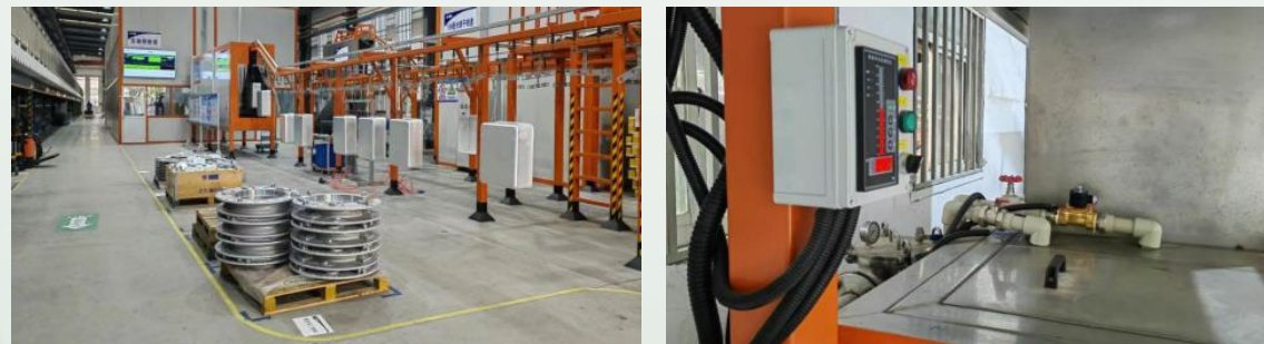
New Powder Spraying Production Line Equipment
